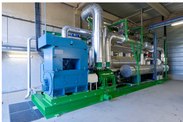
ORCHID© cogen 550 kWe / 4800 kWth, SERM, Montpellier, France
