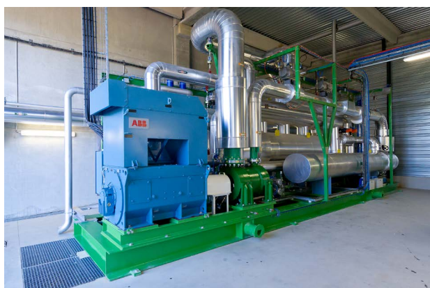
ORCHID© cogen 550 kWe / 4800 kWth, SERM, Montpellier, France
