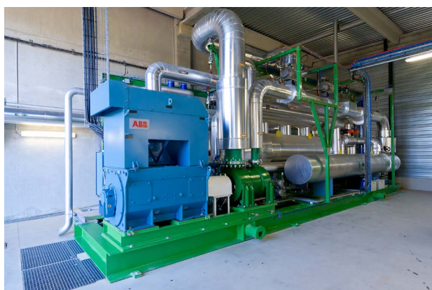
ORCHID© cogen 550 kWe / 4800 kWth, SERM, Montpellier, France
