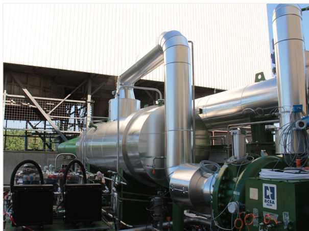
3700 kW Heat Pump on LP Steam, Le Mans, France
