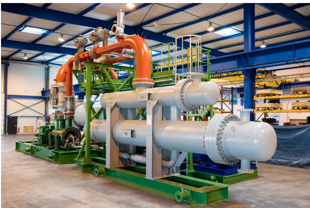
3500 kWe ORC – BaoSteel plant, Shanghai, China
