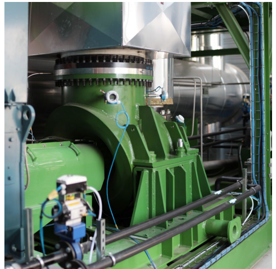
Enertime 2 MWe ORC turbine, Caen, France
