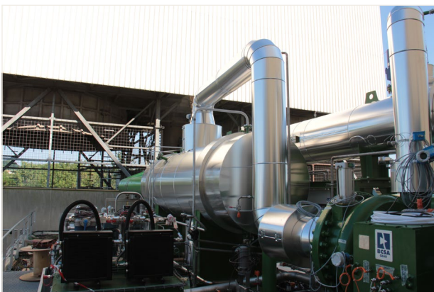
3700 kW Heat Pump, waste incineration plant of Le Mans, France
